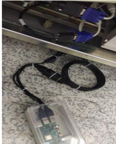
Figure 7. Circuit Design Implemented on Site
